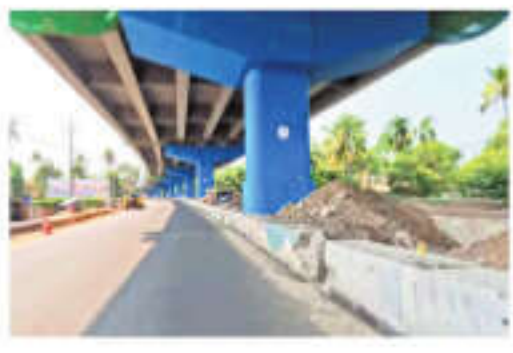
While similar work at the Aroor Bypass Junction has been completed, the remaining work near SN Nagar involves relocating a 110 KV line that crosses the highway
