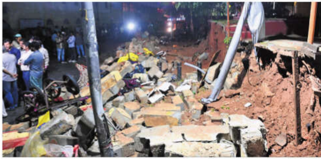
The wall of Bowring and Lady Curzon Hospital that collapsed due to heavy rain at Shivajinagar in Bengaluru on Wednesday | NAGARAJA GADEKAL
