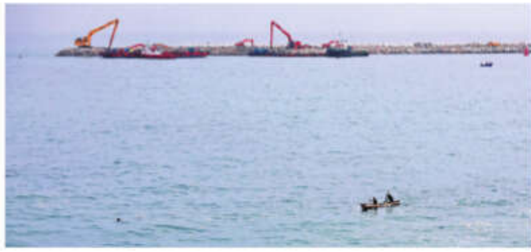
A fisherman rows through the waters off Vizhinjam port as the Phase-II construction work progresses at a rapid pace in the background | ALBIN MATHEW
