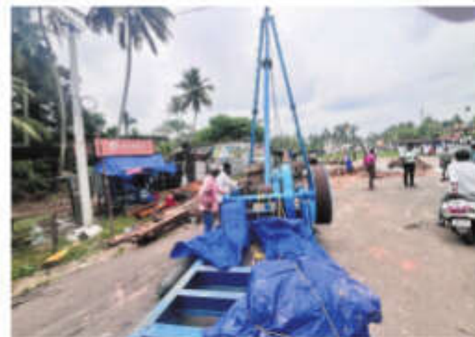
Piling work for Kavalam-Thattassery bridge begins at Kunnumma village in Kuttanad on Wednesday | EXPRESS
