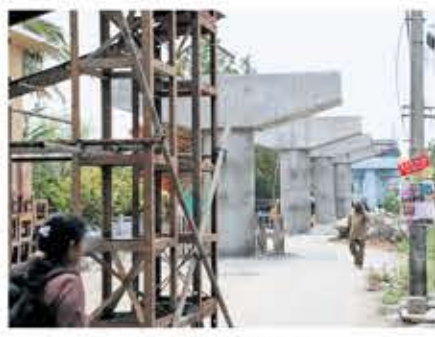
State highways department officials attributed the latest delays to pending utility shifting work | S SENBAGAPANDIYAN
